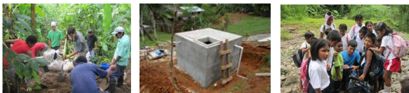
Panama Pictures L-R: (1) EWB members work together to build pediment (2) New Water tank at Centro Sector (3) Bonds grow through community education and outreach
